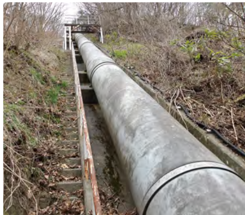
FRP penstock at the Daifudo Hydropower Plant in Aomori Prefecture
