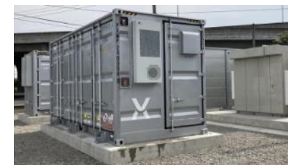
Kozumida Battery Storage Station (Photo courtesy: Bando Battery Storage Station No. 1 G.K.)
