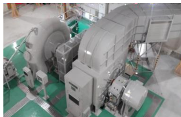
Kidogawa Daiichi Power Station (Hydroelectric)
