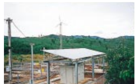
Solar/wind-power generation system with storage battery
